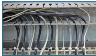
Cable Fixing Cross Members
