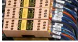
SRS CABLING SYSTEM
