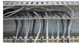
CABLE FIXING CROSS MEMBERS
