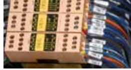
SRS CABLING SYSTEM
