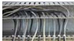
CABLE FIXING CROSS MEMBERS
